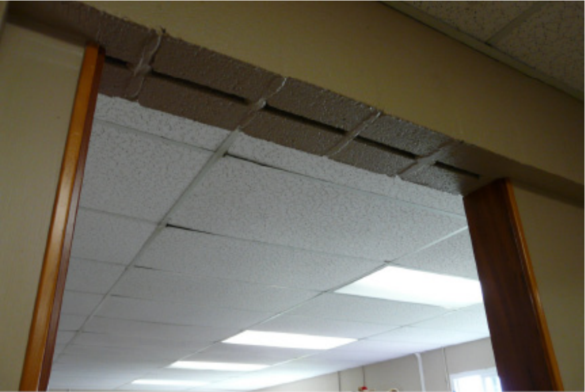
Un-grouted Bond Beam
