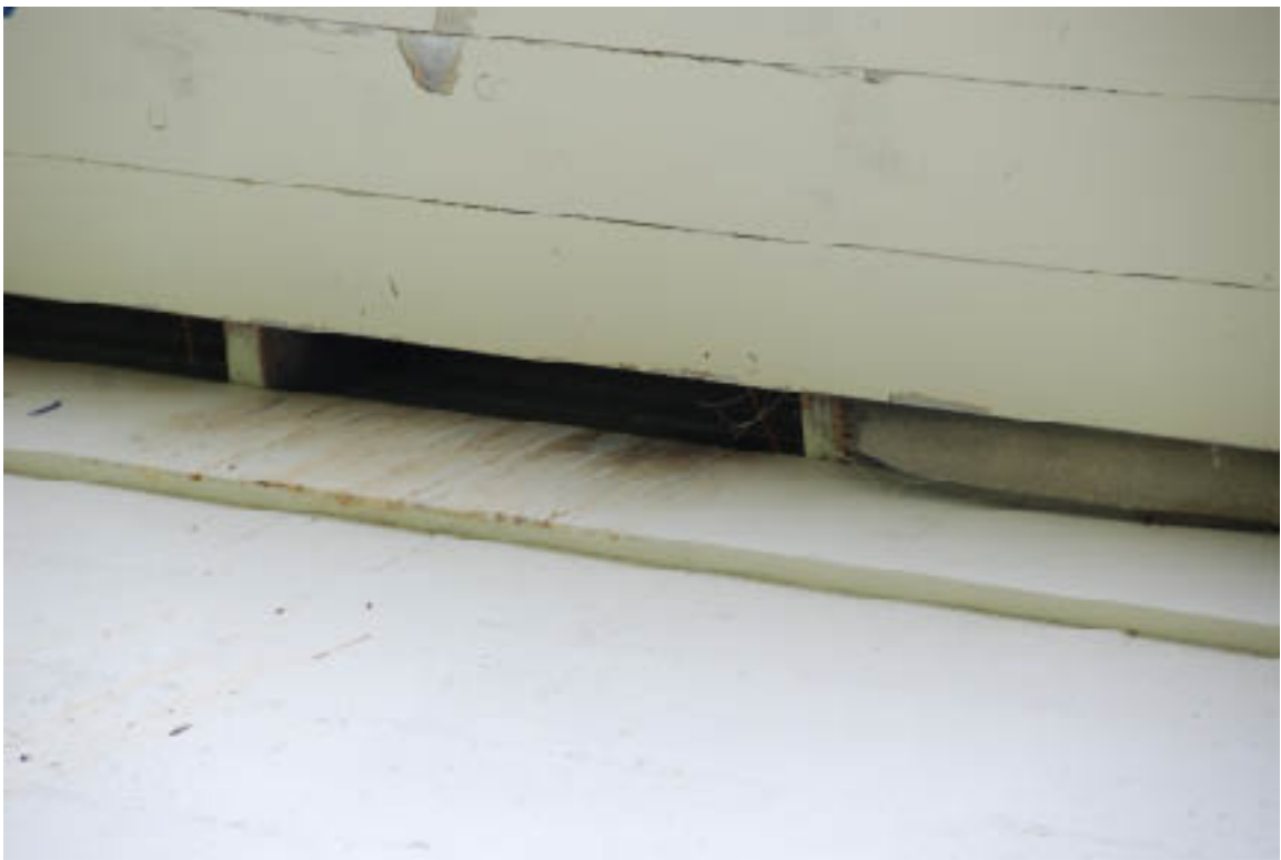
Deteriorated Bird Screen
