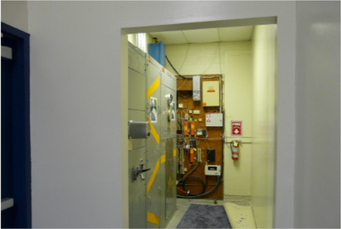
New Main Distribution Panel
