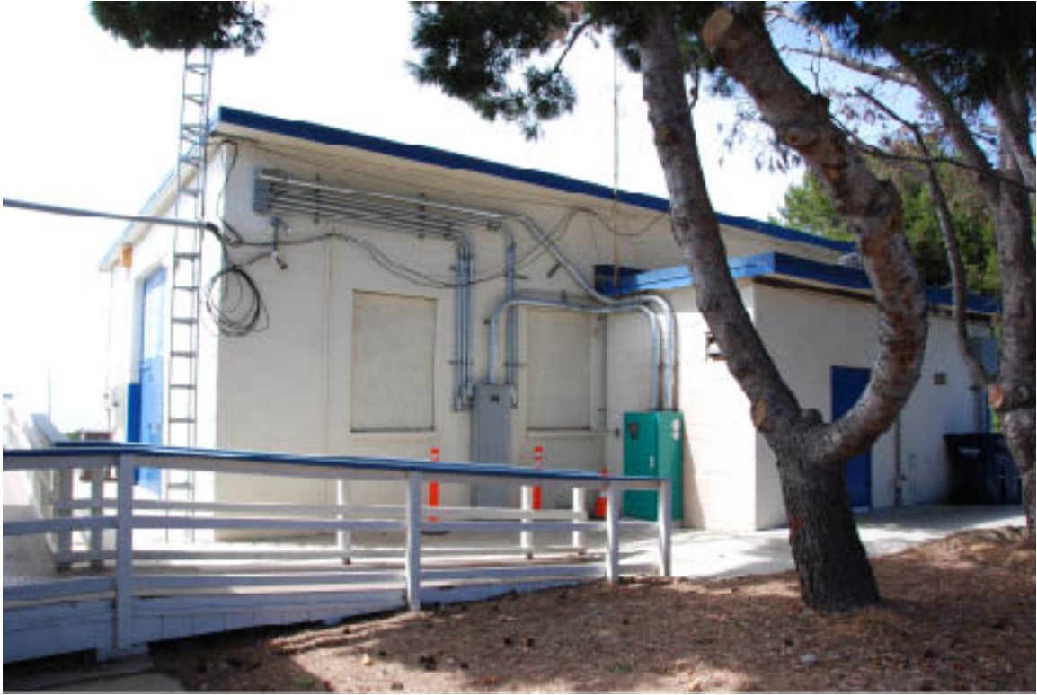
New Emergency Panels
