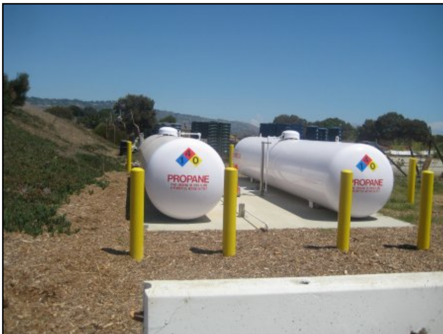
Emergency Generator Propane ATS
