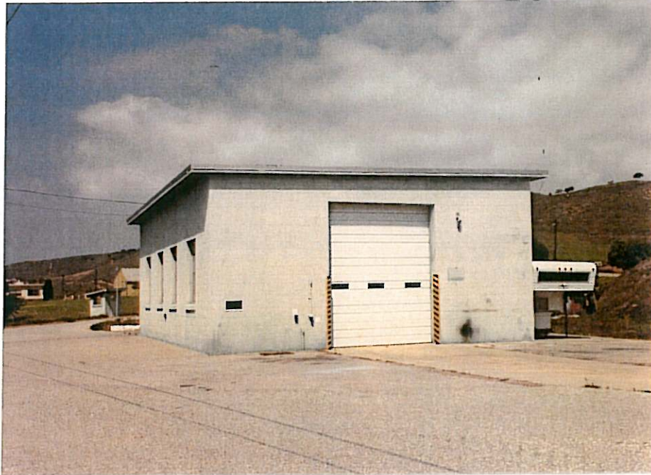
South and west sides of concrete block former fire equipment building near southwest corner of 4.6 acres
