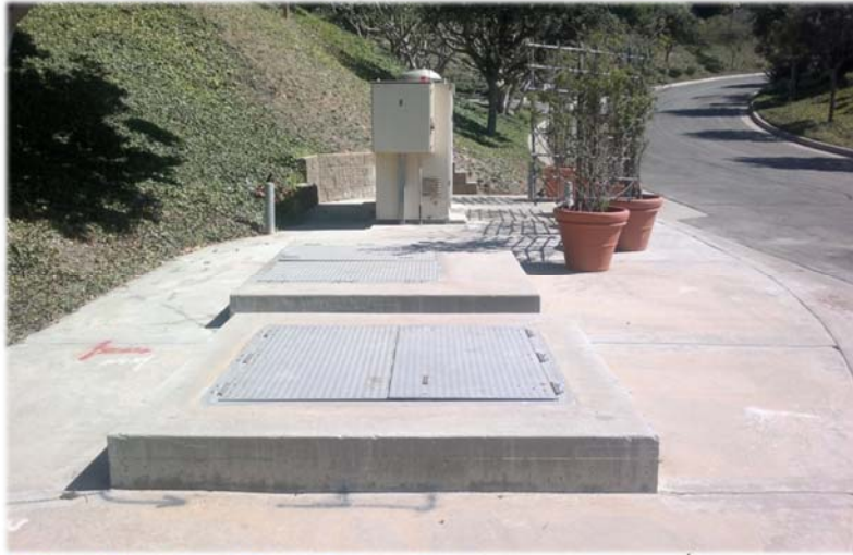
Figure 9.1: Laurel Drive Sewer Station
