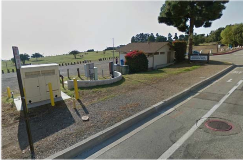
Figure 10.2: Abalone Cove Shoreline Park Sewer Lift Station
