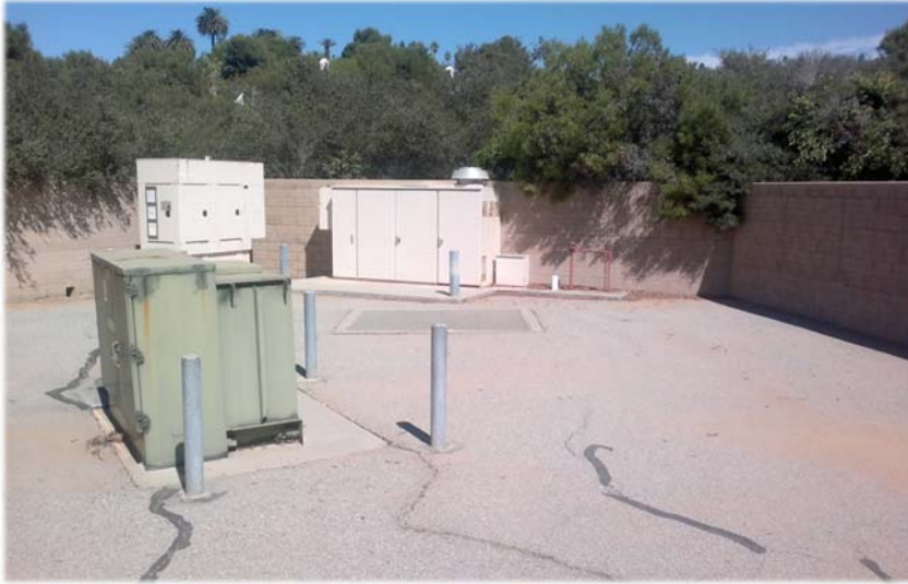
Figure 9.2: Calle Entradero Sewer Station
