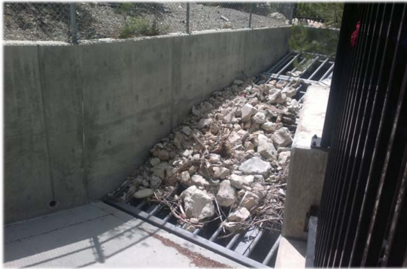
Figure 8.1: McCarrell Canyon Storm Drain Inlet North of PVD South
