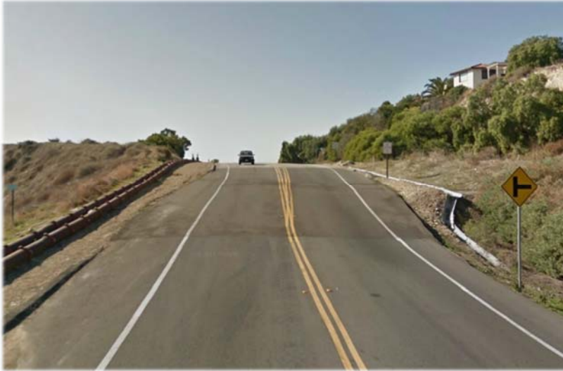
Figure 12.2: Landslide Damage to Palos Verdes Drive South
